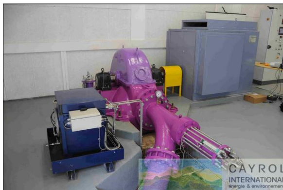
Figure 4 : Turbine Pelton – Centrale de Nohèdes
